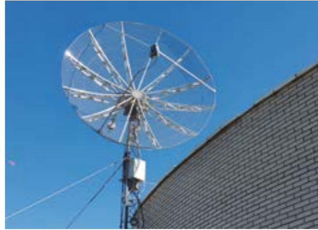
Figure 4: Detail of the Montsec Satellite Ground Station (SGSMontsec), located at the Montsec Observatory (OdM). Credit: IEEC.
