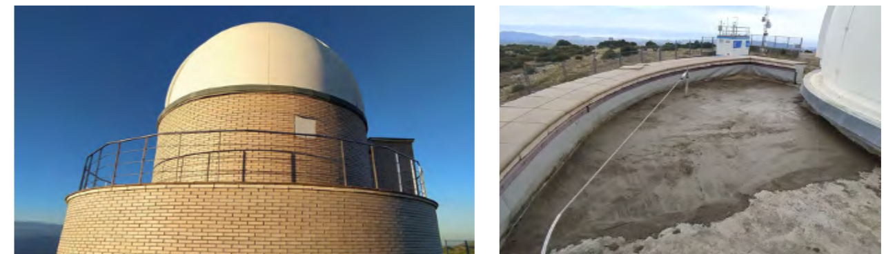
Figure 3: Railings (left) and lifelines (right) installed on the roof of the TJO building.
