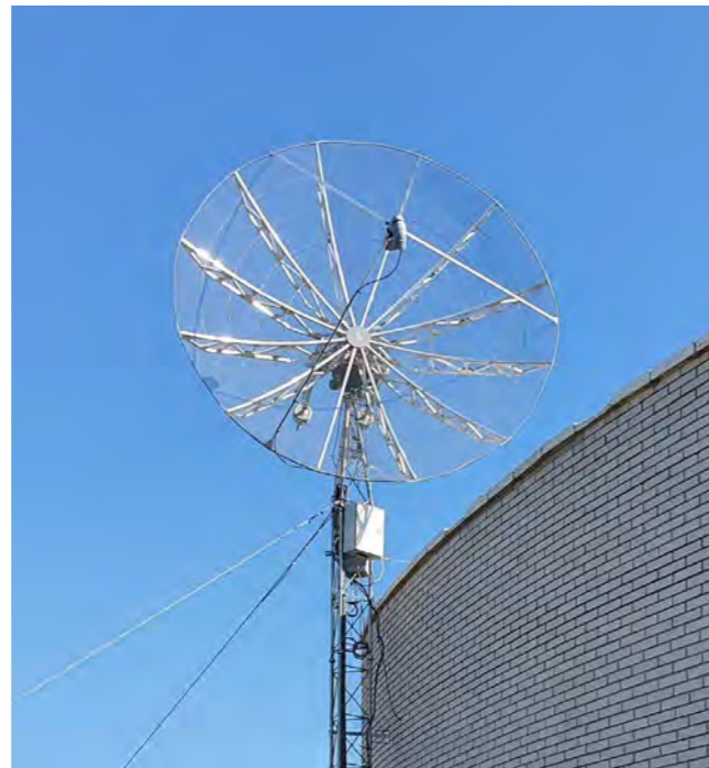
Figure 8: S-band antenna of the SGSMontsec.
